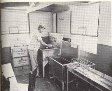
WASHING BOTTLES. Water Supervisor Hienbaugh demonstrates use of motor-driven brush used as first step in cleaning returned empty bottles. High standards of cleanliness and efficiency are maintained throughout bottling plant
